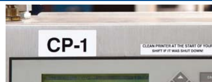
Control Panel & Electrical Panel Labels
