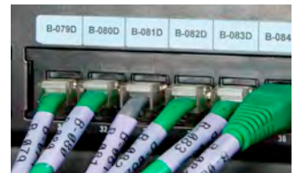
Patch Panel Labels
