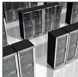
Data Center Servers
