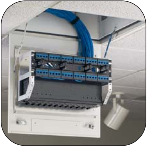
Zone Cable Boxes
