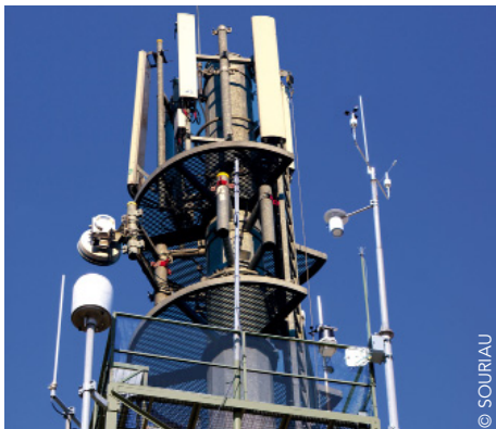
Fiber to the Antenna
