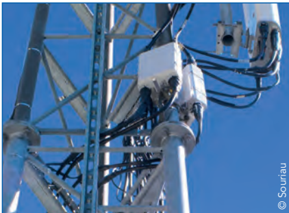
Cell Tower Distribution Box
