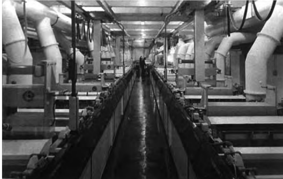
Tyco Electronics' industrial electroplating facilities is one of the most advanced in the world.
