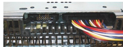
Figure 14 - Control cable plugged into the J1 connector
